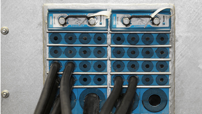
Figure 6. Several types of rodent and fireproof sealings and systems for cable and piping transits are available that ensure a fire proof, airtight, and water-tight transfer.
