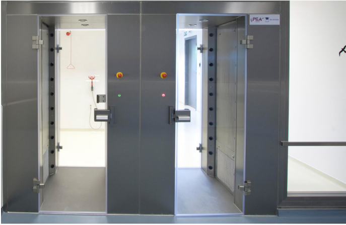
Figure 2. Two air showers built in between the gowning area and a barrier unit.
